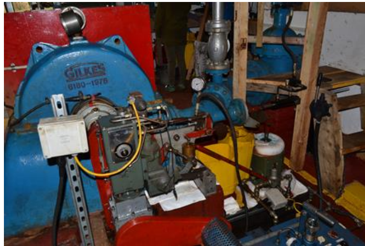
Figure 2 : Generation control system of the present hydro generator which uses a mechanical governor
