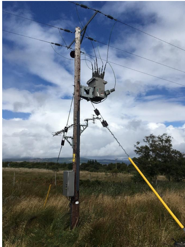
Figure 8 Garmony hydro's pole-mounted transformer
